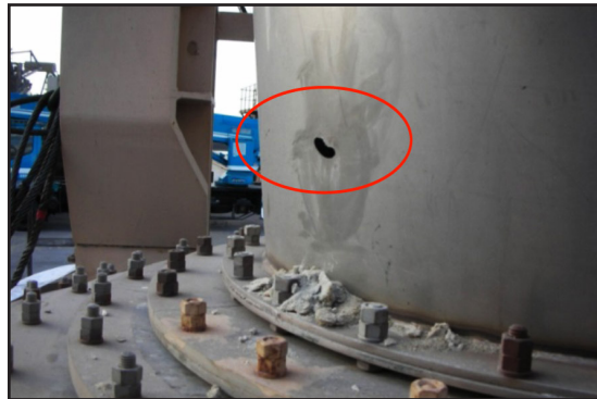
Granulated slag creates holes in the loading chute
